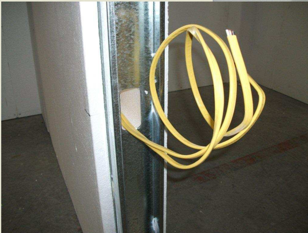
Electrical wiring inside chase
