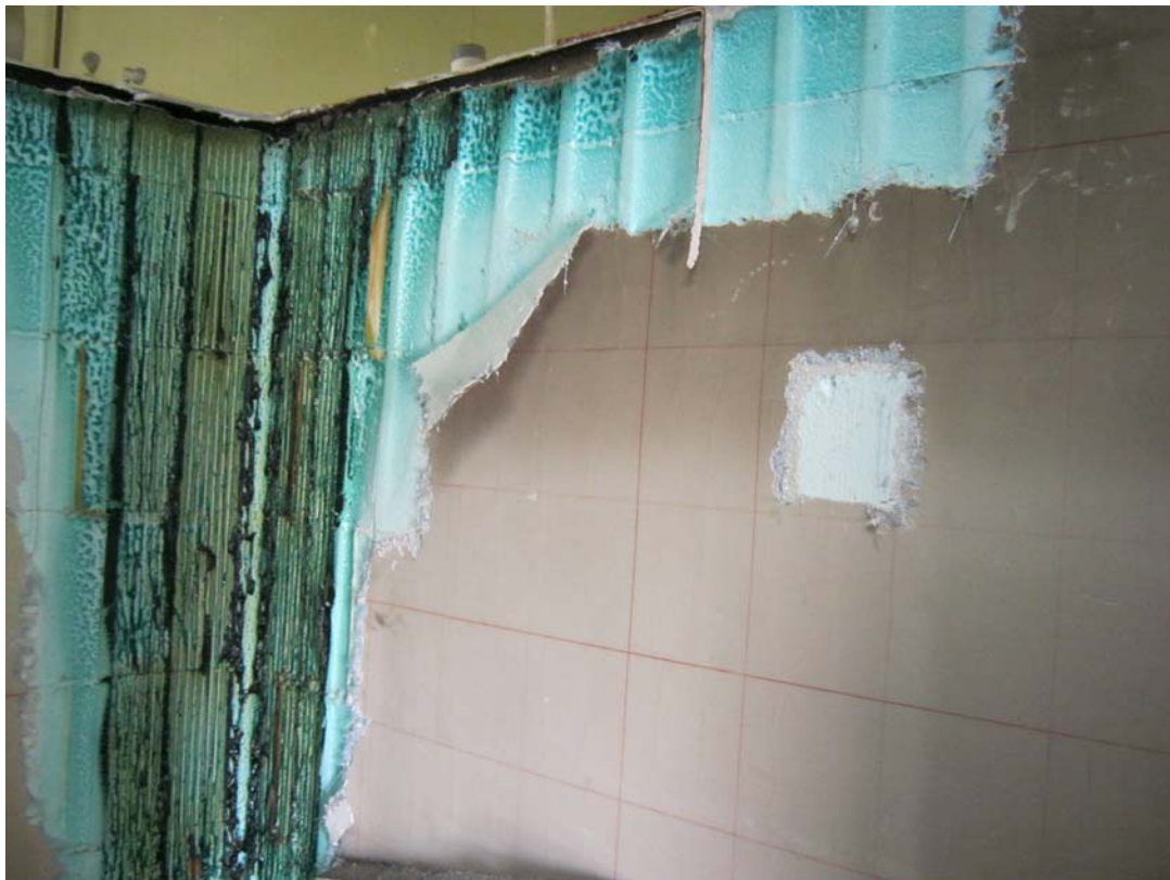
Post Test Photo with Plaster Removed
