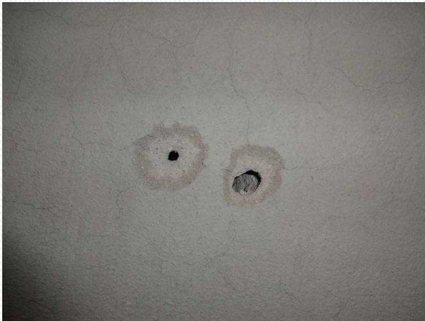
Typical American Portland Cement based 3 coat stucco Over cement block construction, AK-47 shots
